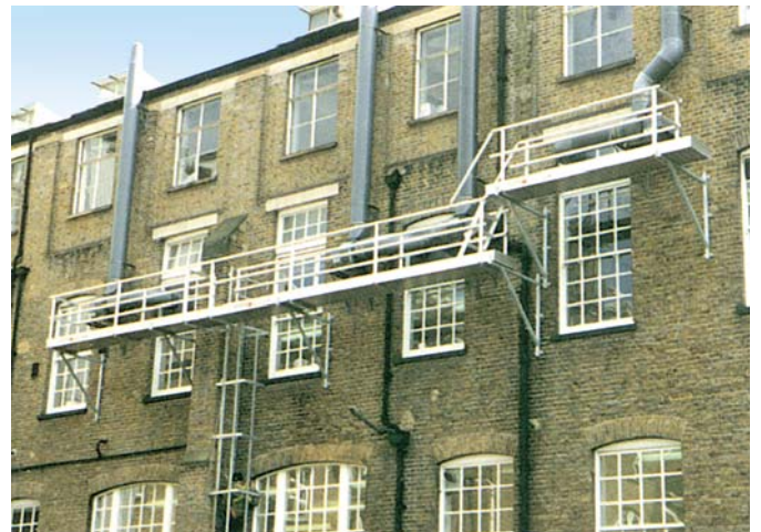
Wall bracket mounted access to soil pipes above busy thoroughfare - City College, London.
