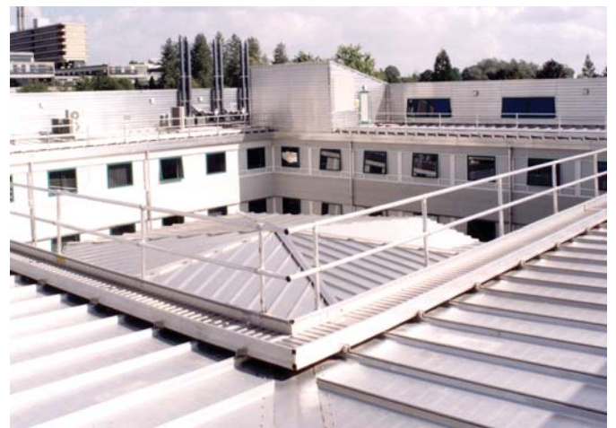
Access over profiled roof to air conditioning plant - Bath University.
